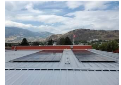
Figure 1 – Solar PV System on the Town Fire Hall
